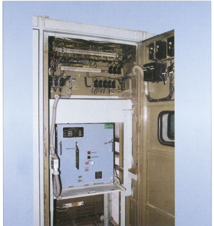
Fig.:2 'Jyoti' Cassette type VCB Draw-out unit
