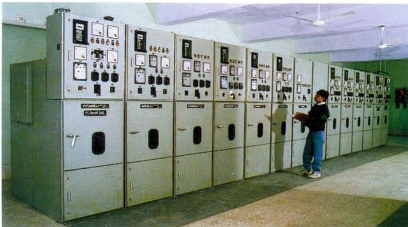
12 kv VCB Panel Installation
