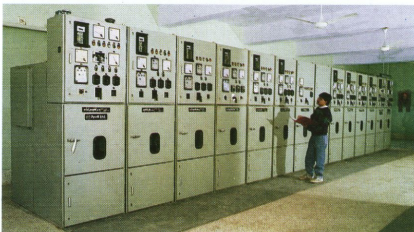
12 kv VCB Panel Installation
